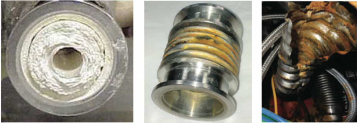
FIGURE 1. Consequences of byproduct condensation in process exhausts; left: solid ammonium chloride blocks an LPCVD silicon nitride process exhaust; middle: flexible stainless steel bellows perforated by corrosive by-product condensate; right: flexible stainless steel bellows ruptured by detonation of reactive solid condensate.
