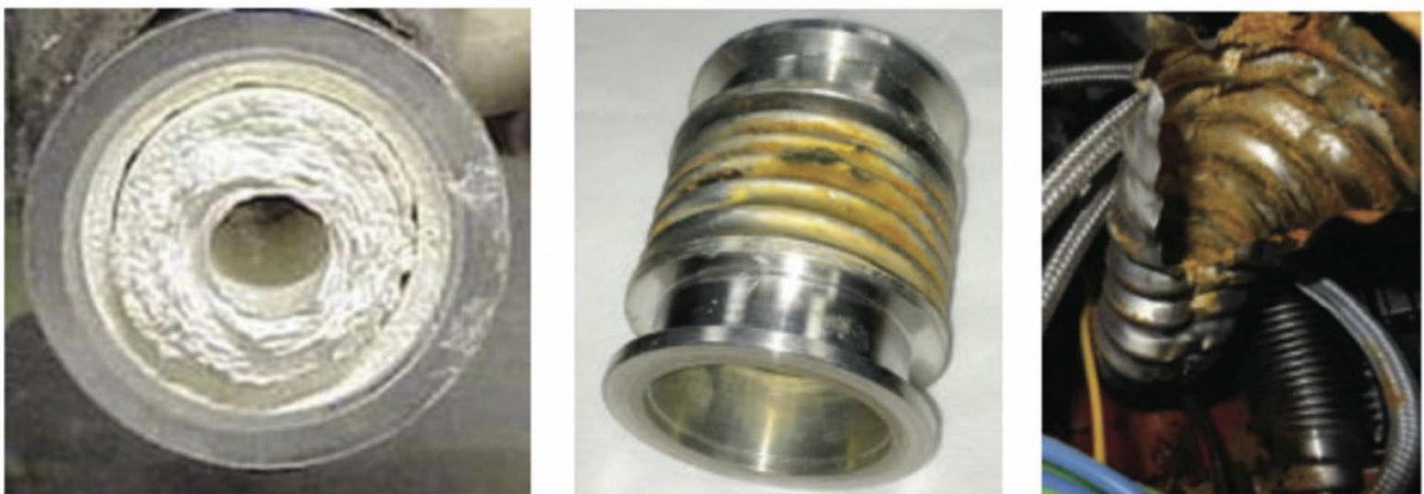
FIGURE 1. Consequences of byproduct condensation in process exhausts; left: solid ammonium chloride blocks an LPCVD silicon nitride process exhaust; middle: flexible stainless steel bellows perforated by corrosive by-product condensate; right: flexible stainless steel bellows ruptured by detonation of reactive solid condensate.
