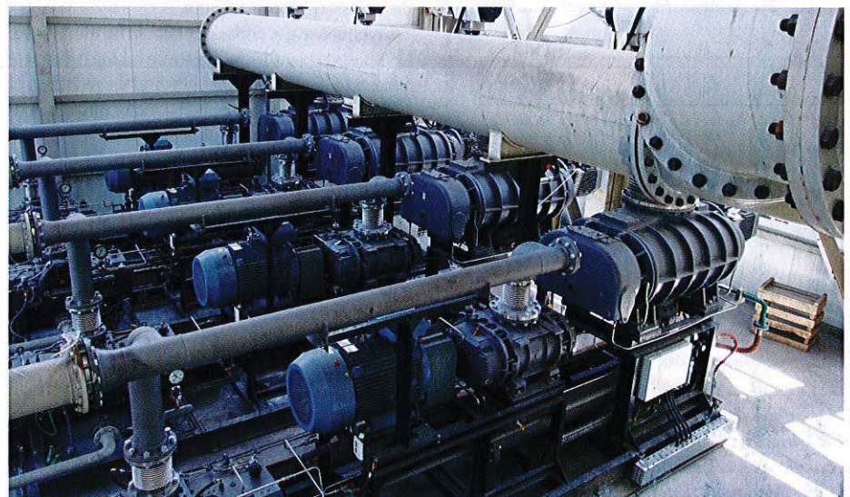
Fig 4. Typical modular dry mechanical vacuum installation for 90 tonnes VD.
