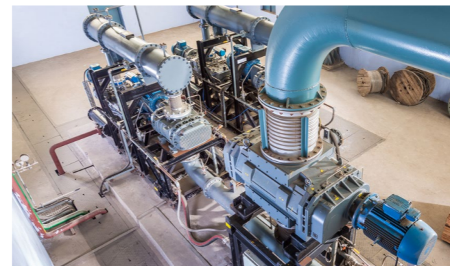
▶ Steel degassing installation FLEXX for VOD
