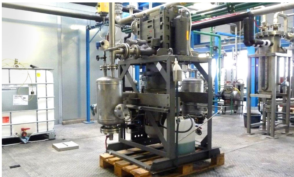
EDP250 with accessories installed at a German polymer producer
