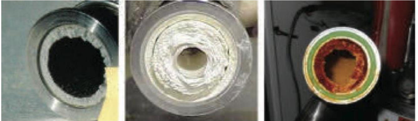
FIGURE 3. Exhaust blockage caused by various materials (left) \text{AlCl}_3 from a metal etch process, (middle) \text{NH}_4\text{Cl} from an LPCVD process, (right) Unknown material deposited in the exhaust of a metal carbide CVD process.
