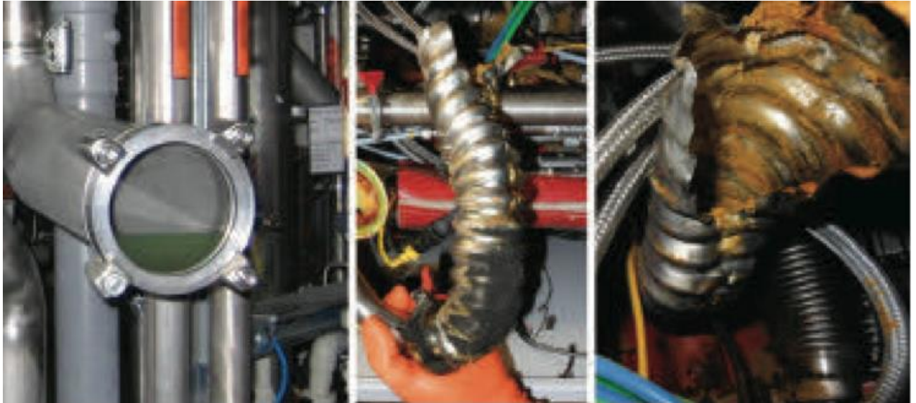
FIGURE 1. (left) Condensed explosive polysiloxane material in an epitaxial deposition system process foreline, (middle and right) CVD exhaust pipe destroyed by explosion of condensed process by-product.
